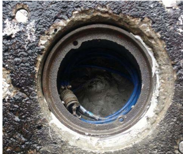
Figure 13. Hole OC-4 temperature probe and flush-mount cover photos.
