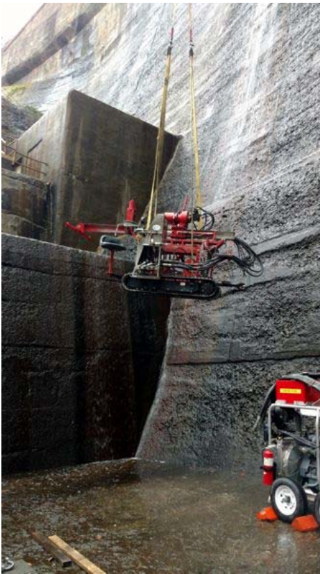
Figure 7. Accessing the toe of the dam using rubber-tired vehicles and cranes from the top.
