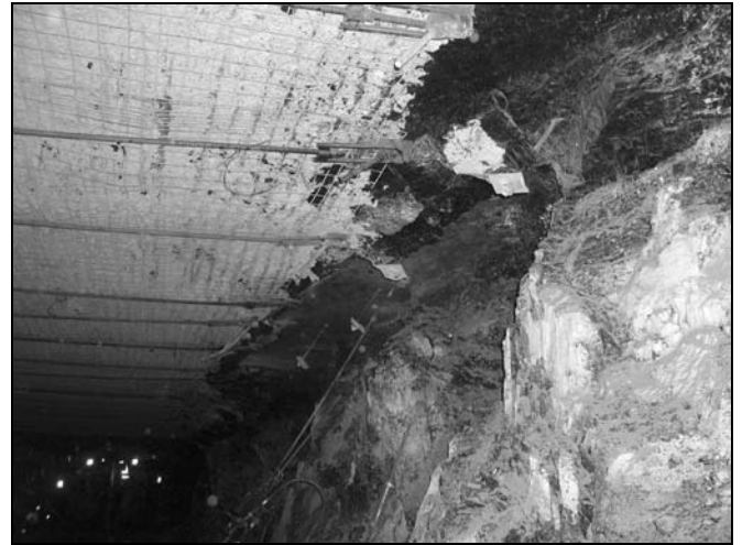
Figure 9. Horizontal Stress Damage Along Corner of Roof
