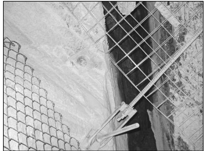
Figure 10. Open (15 cm) Aperture along Fault Blade in Roof in Low Horizontal Stress Zone
