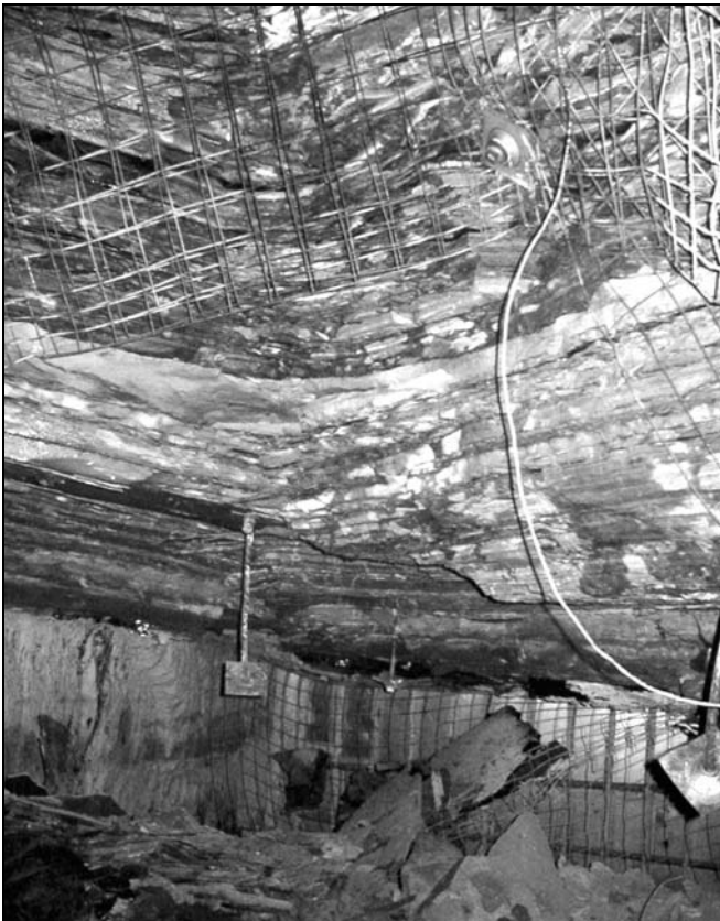
Figure 8b. Horizontal Stress Damage in the Roof—Roof Fall Following Crushed Zone
